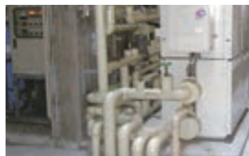
■ Bathroom heating system with filtration unit
